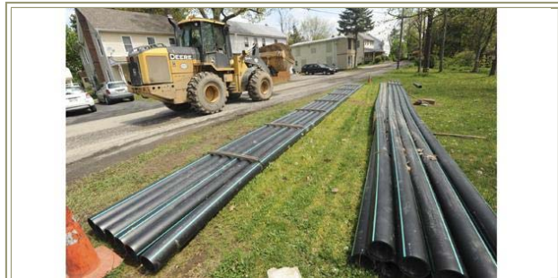
New sewer lines are going in through Cairo's business and residential district, upgraded from the smaller piping originally installed over 10 years ago. The improvements will help solve problems experienced over the years due to undersized lines that affected service. Here, new lines await installation on Grove Street. Photo by Claude Haton
